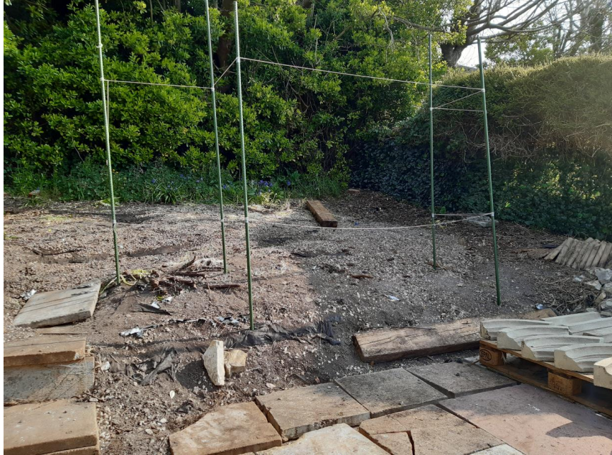
Area of proposed folly with mock up showing the level of the raised platform (lower string) and the top of the structure (higher string).
